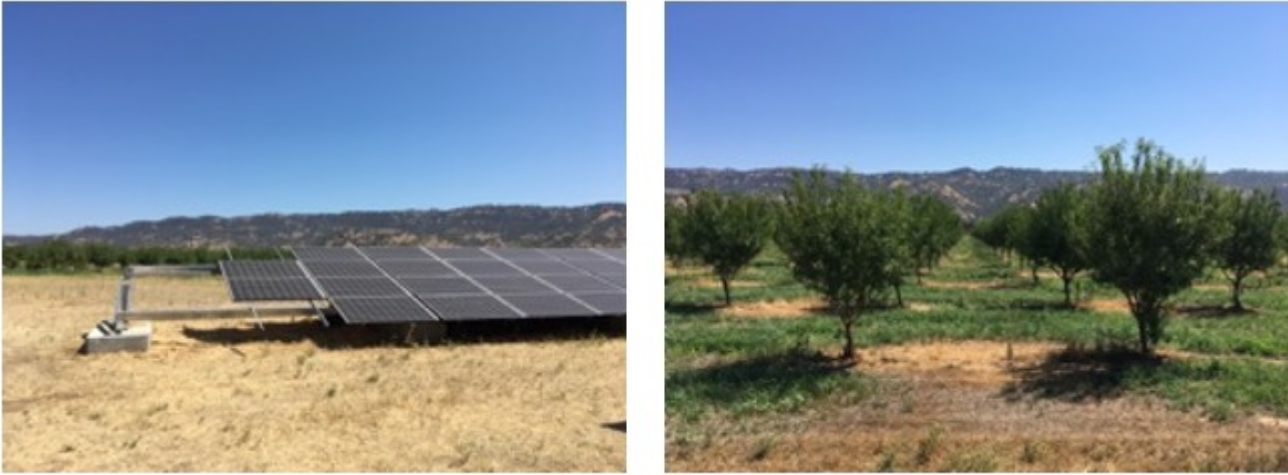
Image 7: Solar panels were installed at Full Belly (left) to irrigate a new 12-acre almond orchard (right).
